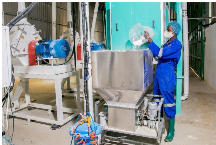
USAID Advancing Nutrition. A production personnel at Njojo Agro-based Industries demonstrates how the dosifier installed after training on food fortification is used. Photo credit: USAID Advancing Nutrition.
